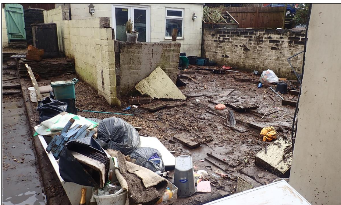
Figure 6: Damages left after the event to the rear of a property at Cilfynydd Road captured by FRM officers on 17 th February 2020
