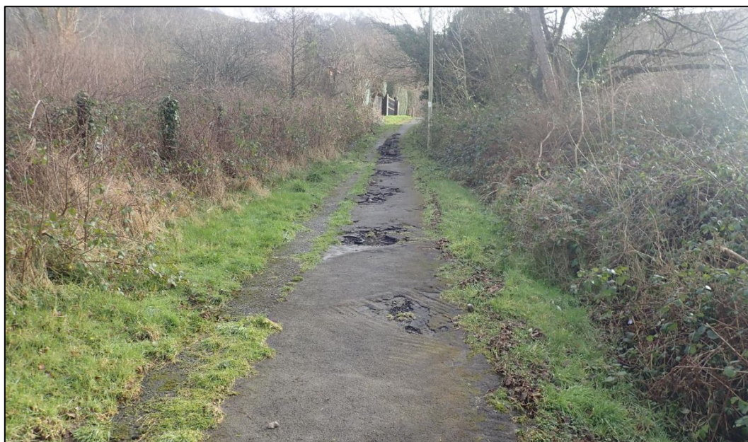
Figure 11: Evidence of damages to the top of the path looking up towards Heol Nant (captured by FRM officers on 17 th February 2020)
