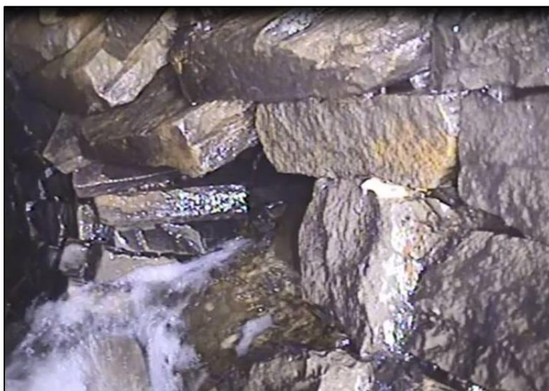
Figure 20: Hole in culvert 22.9 meters downstream of the Ely Brook inlet opposite Royal Oak Inn
