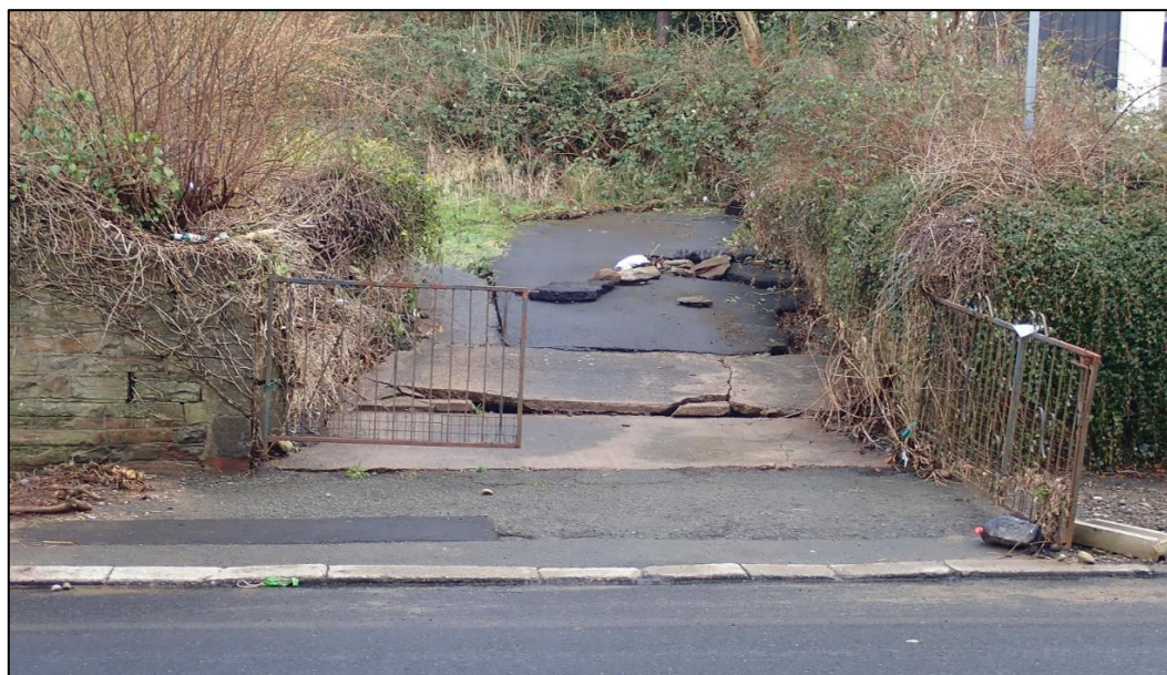
Figure 14: Damages to the driveway situated below the Ely Brook culvert inlet showing evidence of subterranean hydraulic pressure (captured by FRM officers on 17 th February 2020)
