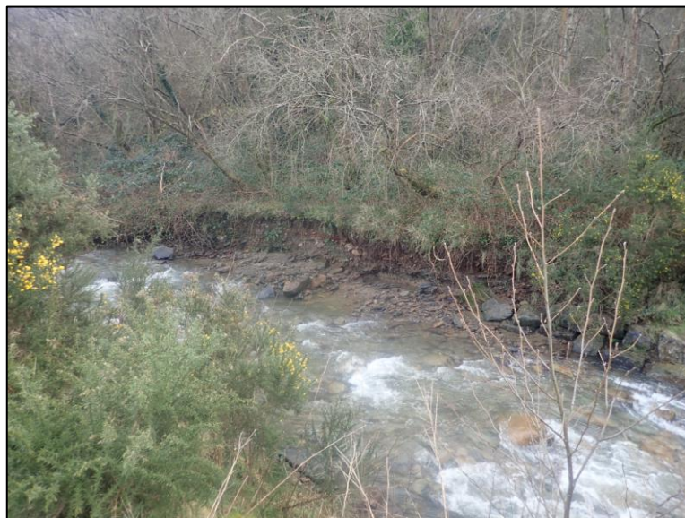
Figure 27: Photo of embankment scour to the Nant Cae Dudwg watercourse (image captured by RCT's Flood Risk Management team on 02/03/2020)
